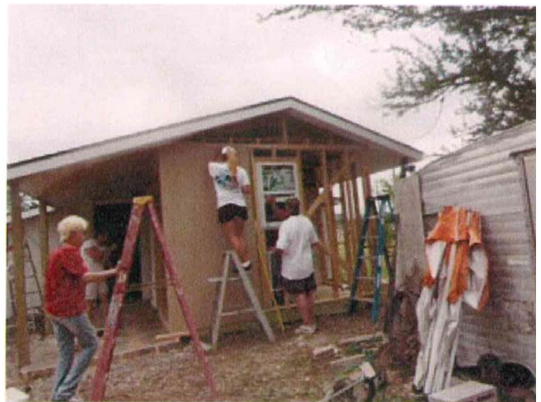
Added a utility room at to a Church ladies small house by Azle Mission work group 2017.
